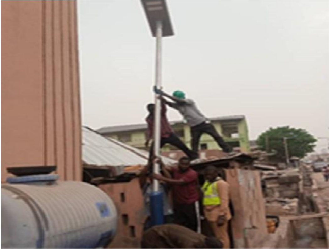
COMMUNITY DEVELOPMENT SCHEME: INSTALLATION OF SOLAR STREET LIGHTS AT CENTRE IGBORO COMMUNITY ILORIN SOUTH L.G.A, KWARA STATE
