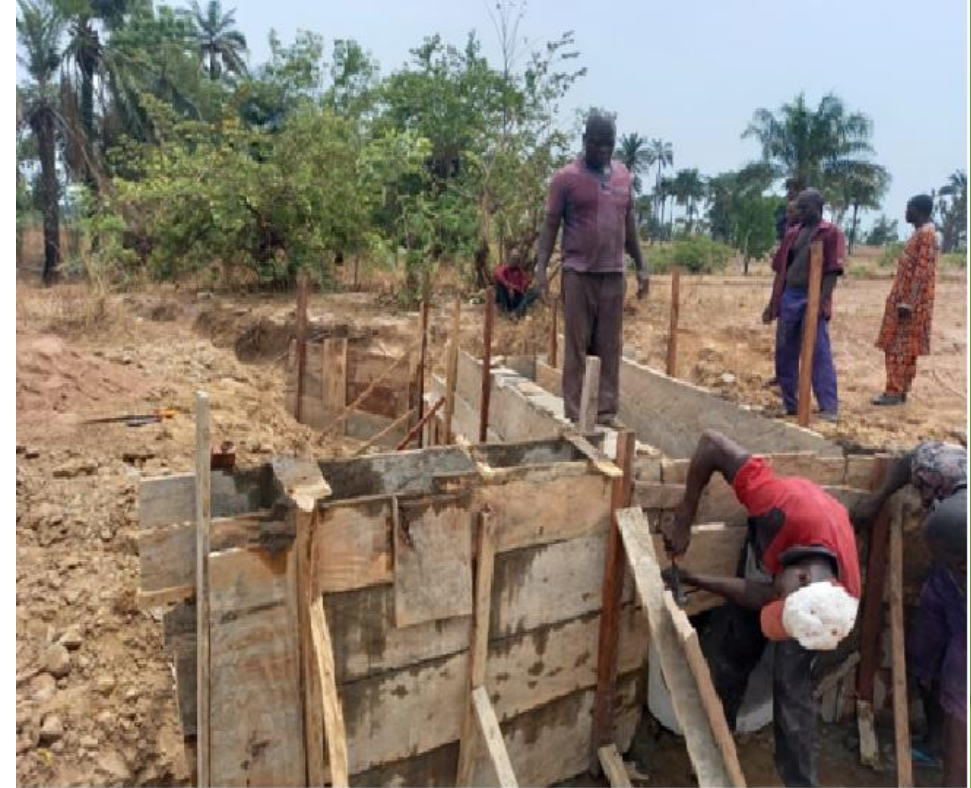
COMMUNITY DEVELOPMENT SCHEME: CONSTRUCTION OF SINGLE AND MULTIPLE PIPE CULVERTS AT BURI AND EKPON 1 COMMUNITIES, NASARAWA STATE
