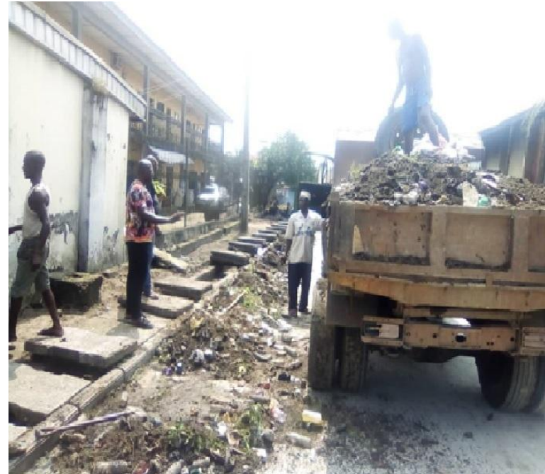
COMMUNITY DEVELOPMENT SCHEME: WORKERS DESILTING THE DRAINS DURING THE CONSTRUCTION OF 100M CONCRETE PAVEMENT ROAD WITH SIDE DRAINS AND COVER SLAPS, EFFURUN, DELTA STATE.
