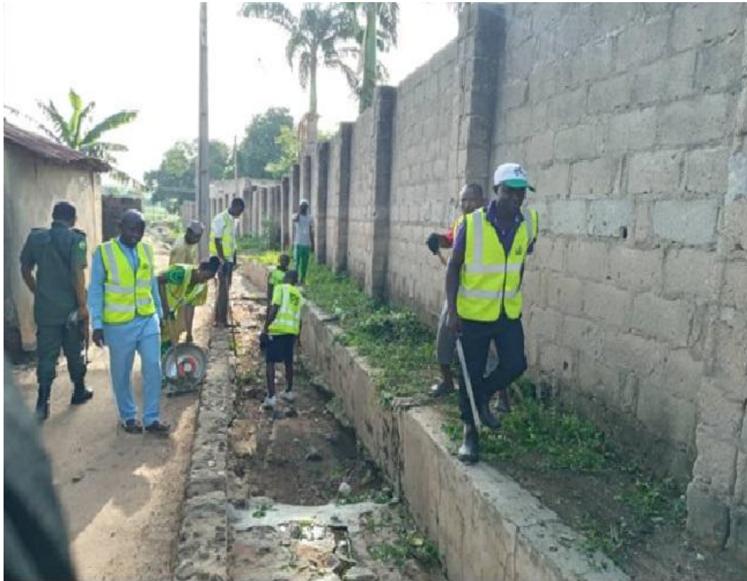
EXTENDED SPECIAL PUBLIC WORKS PROGRAMME (ESPW 774,000 JOBS): DRAINAGE MAINTENANCE AT LAFIA LGA, NASARAWA STATE
